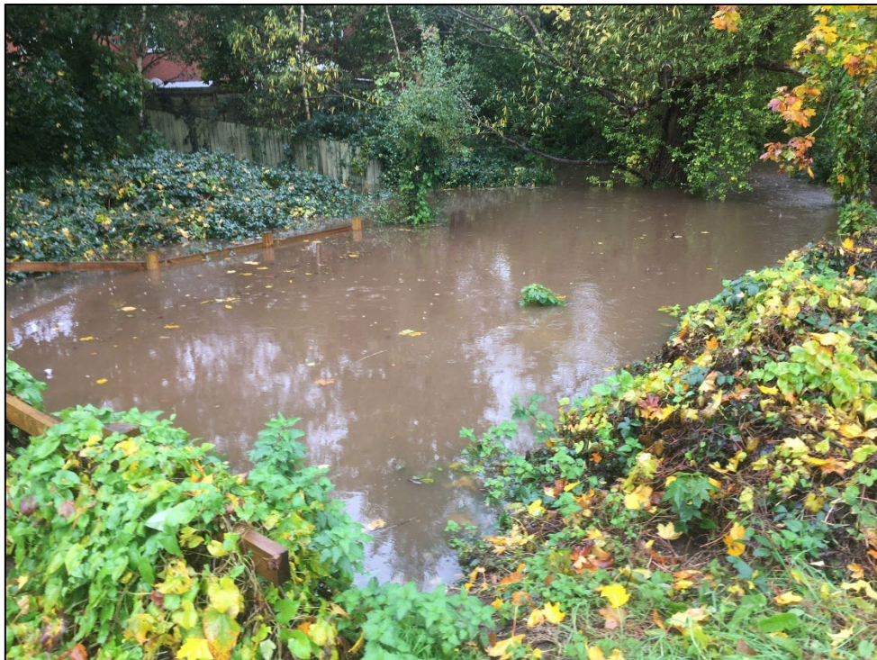
Photo taken during the October flood event looking over the Greenway culvert.
