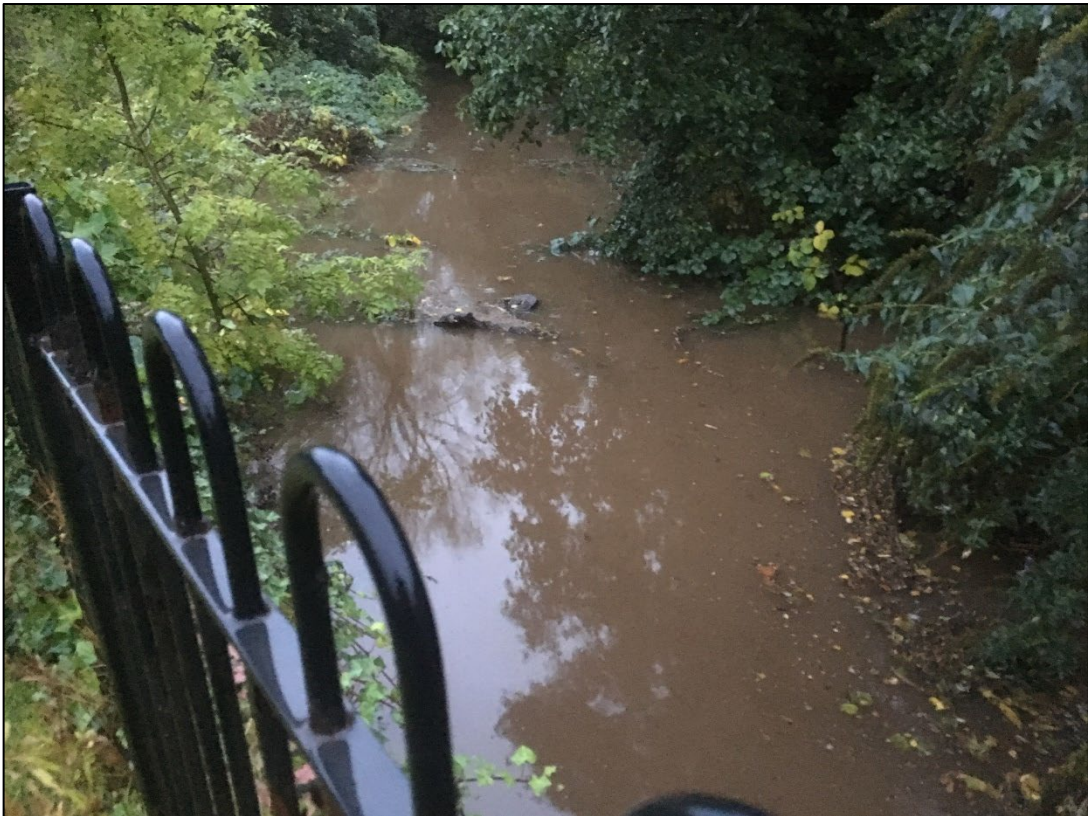
Photo taken during the October flood event looking over the Chestnut Drive culvert towards The Greenway.
