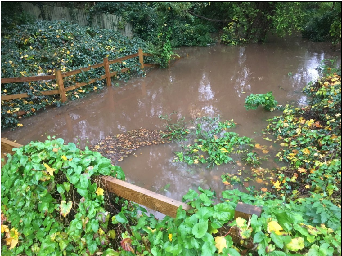
Photo taken during the October flood event looking over The Greenway culvert towards Chestnut Drive.
