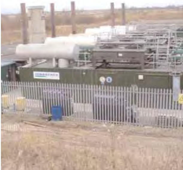
Landfill gas management plant (Hill and Moor Landfill site, near Pershore)
