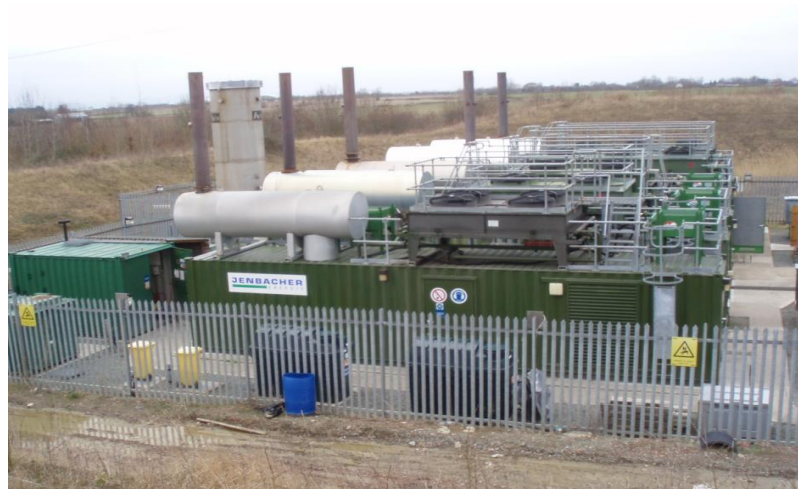
Landfill gas collection at Hill and Moor landfill site, near Pershore, Worcestershire
