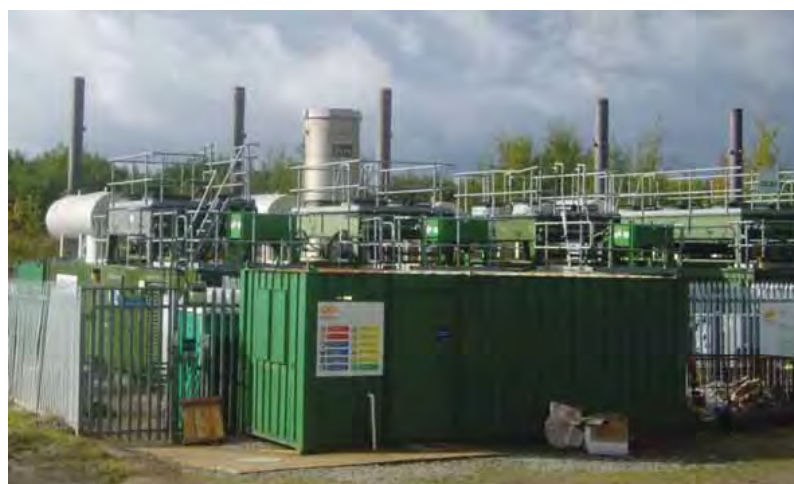
Landfill gas management plant (Hill and Moor Landfill site, near Pershore)
