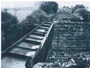
A bridge strike can seriously damage railway bridges
