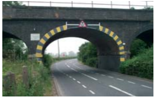
White lines on the road indicating the extent of the signed vehicle height limit
