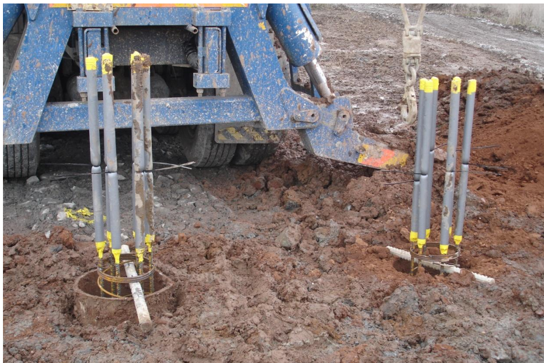
Two piles with the steel cage reinforcement protruding, which will link into the pile cap foundations
