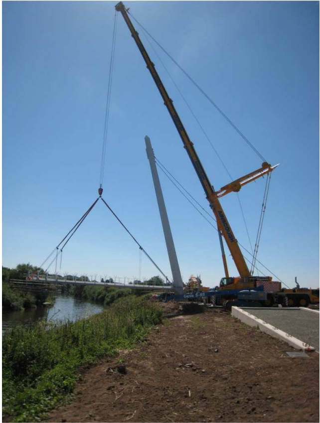
The first 24.5m long deck section being craned into position by the 500 tonne crane
