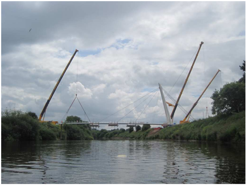
The fourth and final 19.5m long deck section completing the 66m river span
