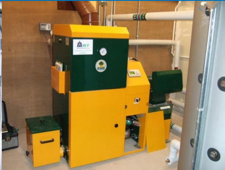
Biomass (wood-chip) boiler
