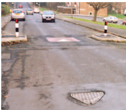
Poor road surface on approach to traffic calming. Keith Sharples Photography.
