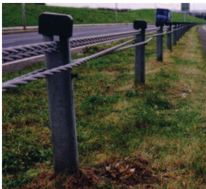
Wire Rope Safety Fence and support posts. Keith Sharples Photography.
