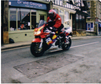
Poorly located utility cover. Keith Sharples Photography.
