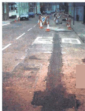
• p16 Patchy workmanship
